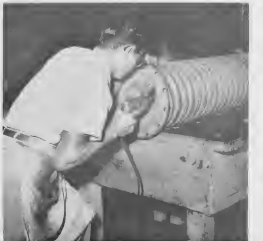
WITH A pistol-grip electric drill, B. Tromp, tradesman B. CU UN drill electrico di mas, B. Tromp, tradesman B, ta drill buraco pa schruof den un expansion joint.
